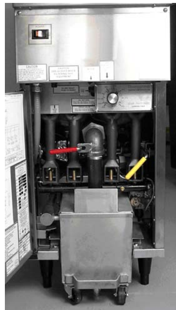
Typical Single Under Fryer Filter (SUFF) installed in a single fryer.
